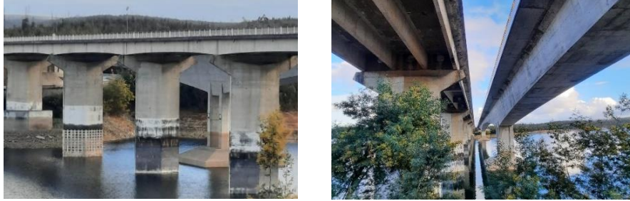
Fig. 1. Bridge over the mouth of the Dão river. Old structure affected by the expansive reactions and, in parallel, the new box girder deck bridge.
