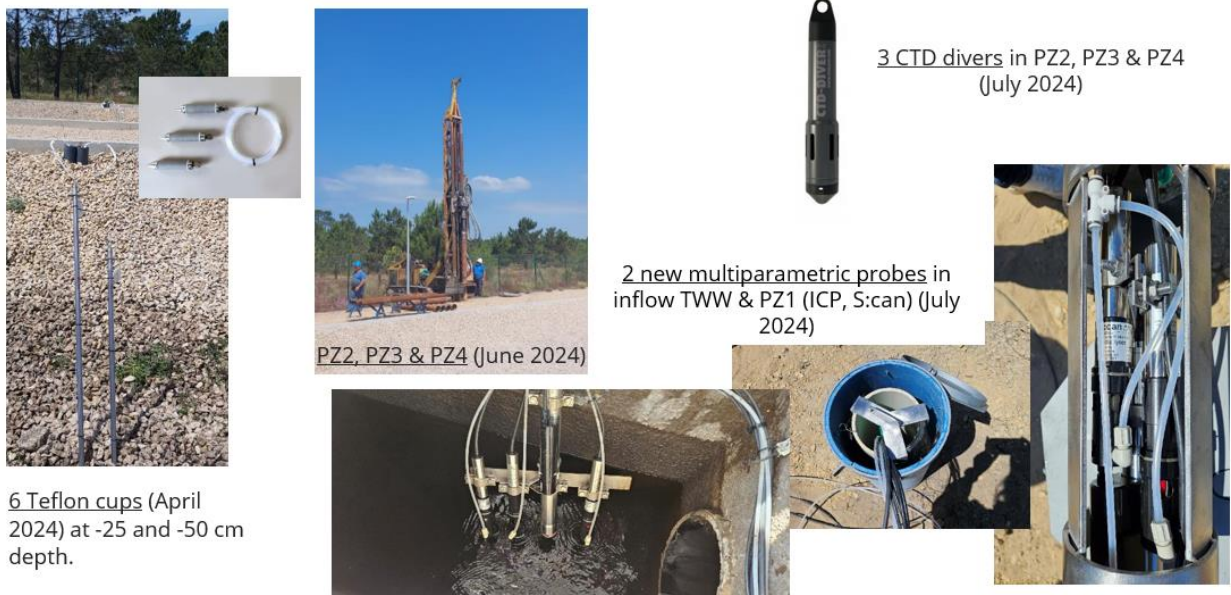
Figure 2.6 Monitoring and sampling equipment installed under MARCLAIMED at Comporta WWTP_SAT-MAR
