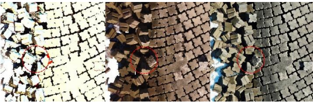
Figure 20. West breakwater. Changes found between 2020 and 2022 – Occurrence 3 – Section G
