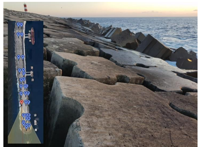
Figure 6. 2018 visual observation at Point 27F (F – Front direction) of Sines west breakwater (outer armour layer)
