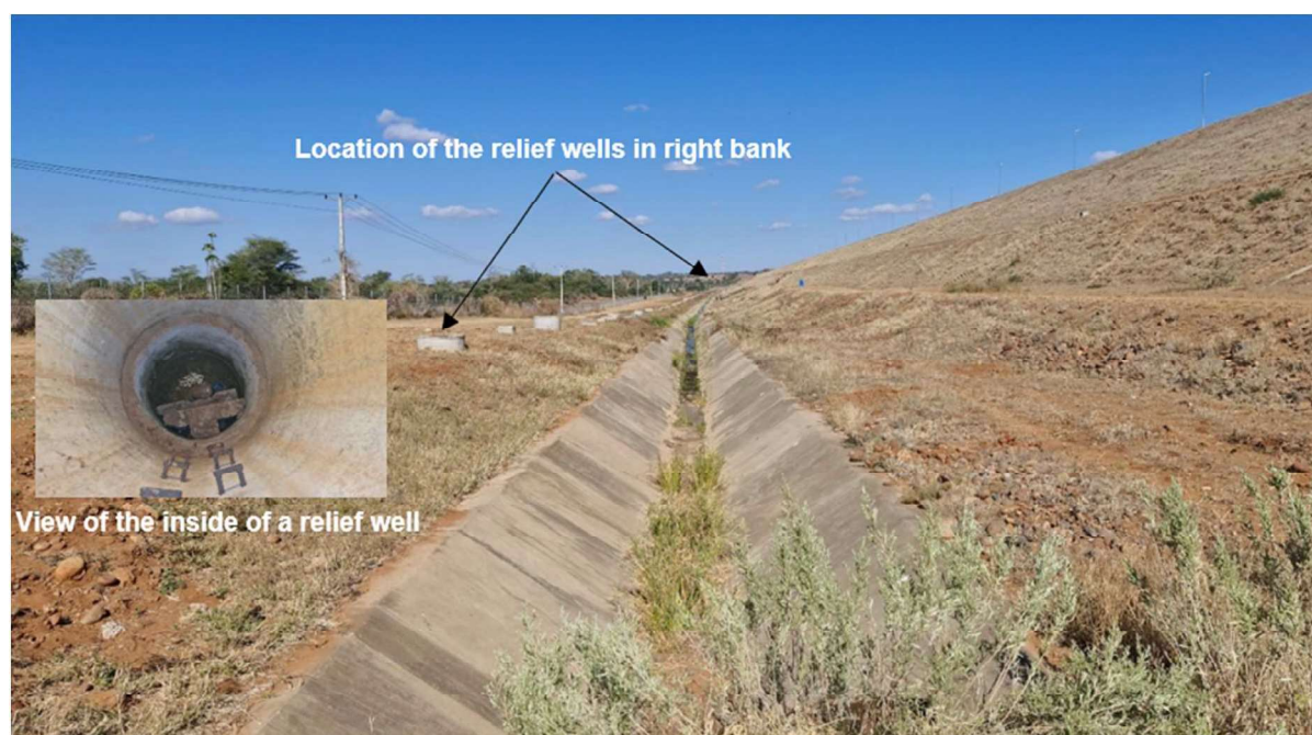
Figure 4 – Relief wells in the right bank
